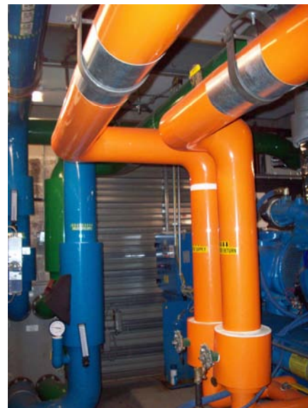
TECOCHILL STx Series CHILLER installed in the Whitman Laboratory in 2007.
